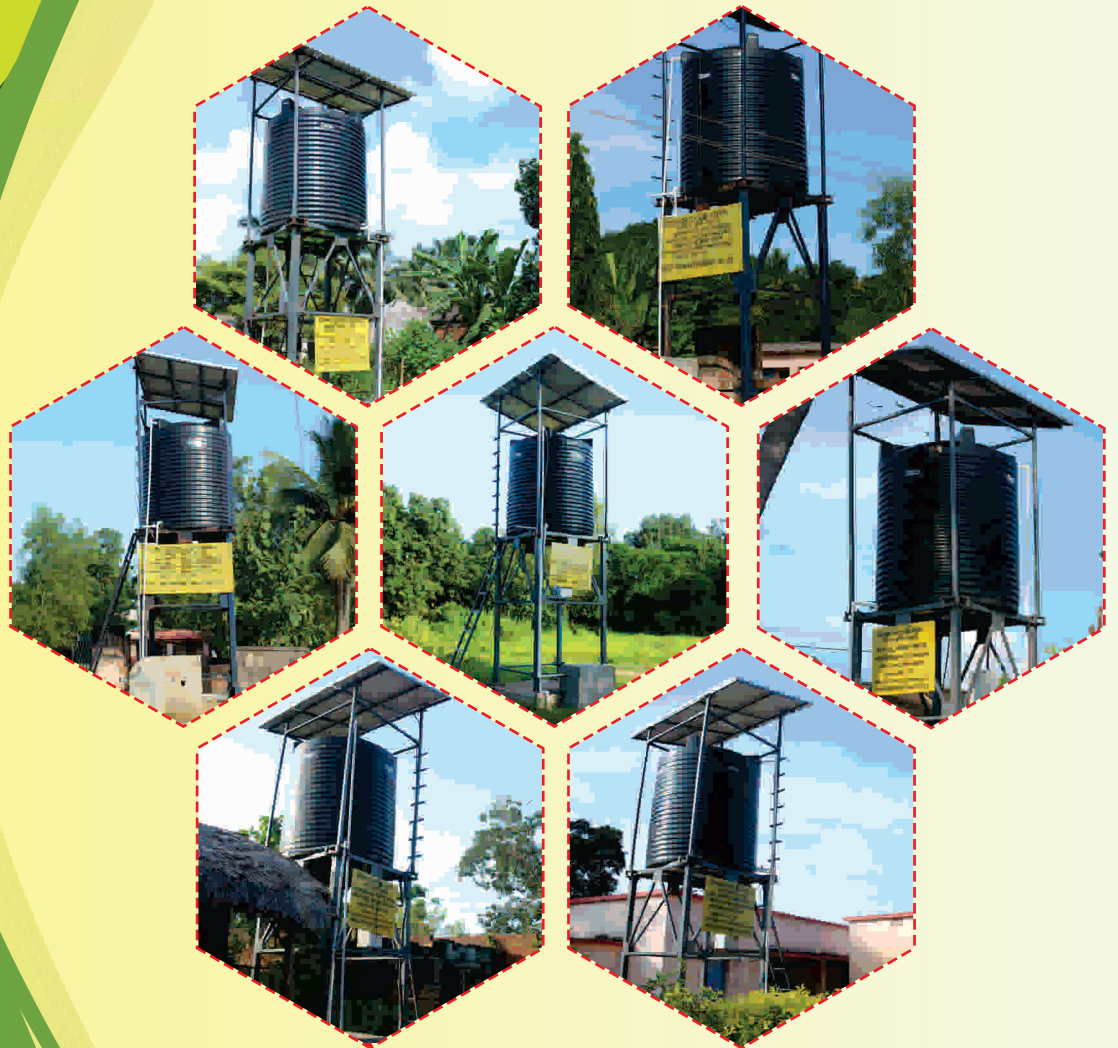
Photo Gallery of Solar based drinking water supply system
